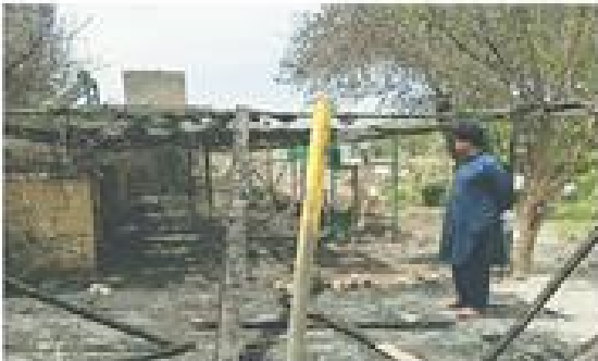
OFFICIALS examine the damaged bridges at the wildlife park in Lakki Marwat. — Dawn
