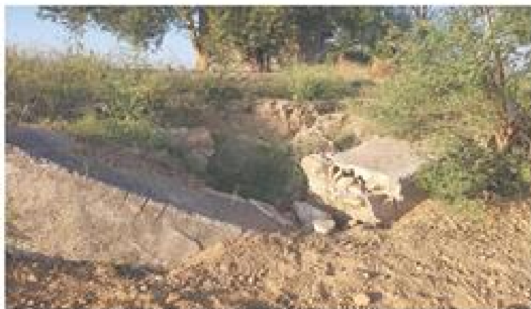
THE retaining wall in need of urgent repair.
