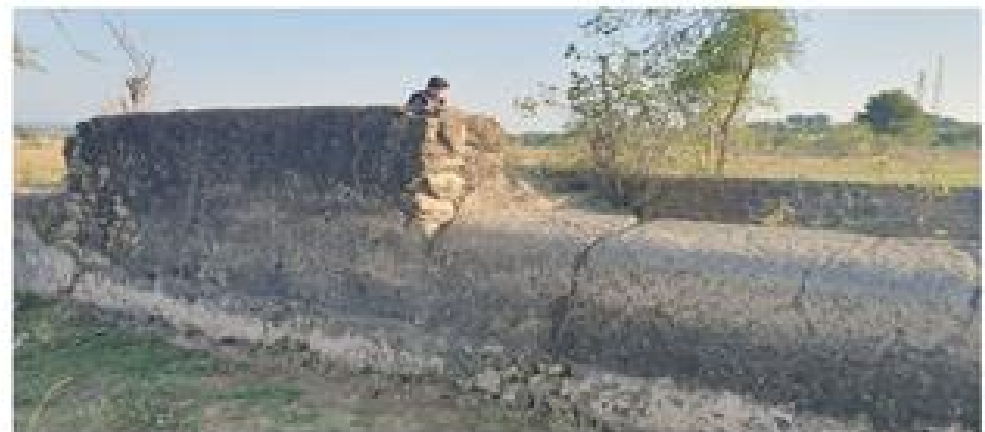
An outer view of the crumbling boundary wall of the Baoli.
