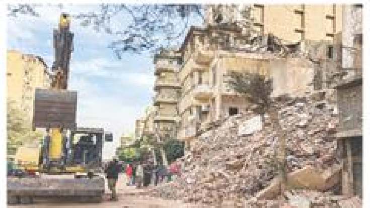
CAIRO: An excavator is stationed outside a collapsed building. Eight people were killed and three more injured in the Egyptian capital on Tuesday when a six-storey residential building collapsed.—AFP
