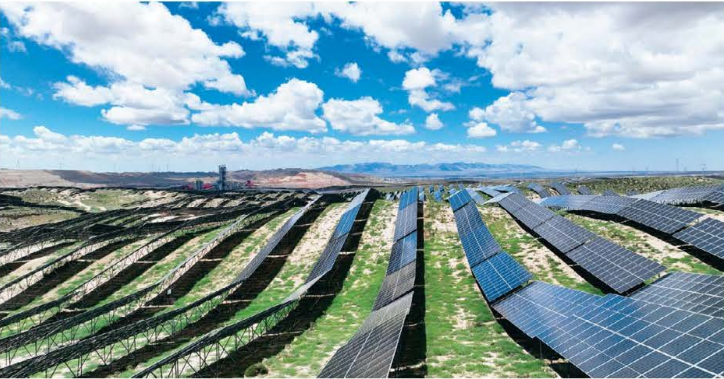
A solar power station in Ningxia Hui autonomous region. China's photovoltaic industry is struggling with overcapacity. Photo: Xinhua
