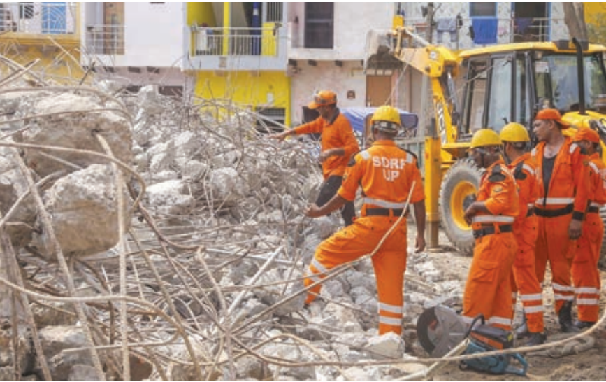
Rescue work underway after an overhead water tank collapsed on Sunday in Mathura. At least two women died and 11 people were injured after getting buried under the debris of the tank, according to officials.
